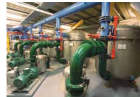
FILTRATION EQUIPMENT AIS
